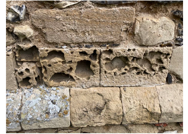
Alveolar Weathering / Wind Scouring Example at Leiston Abbey
