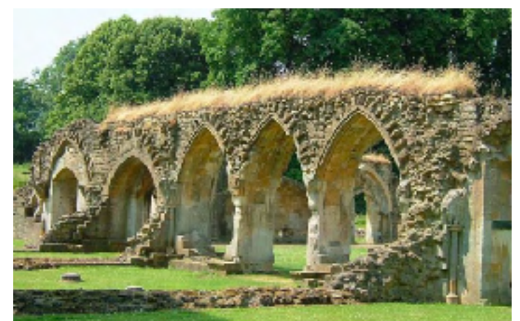
Soft Capping to a historic ruined wall at Hailes Abbey in Gloucestershire
